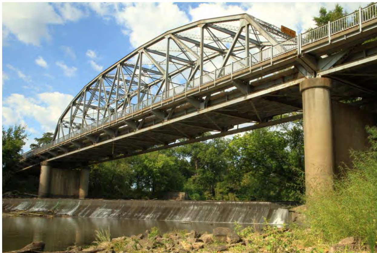
Figure 3. Photograph of the low-head dam at OK-123 along the Caney River (ODOT, 2016)
